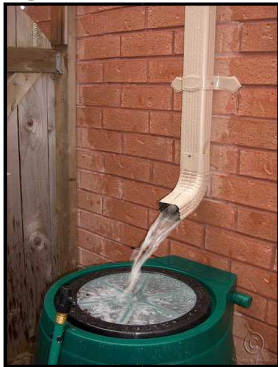
Figure. 4 Rainwater collection (through downpipes and sieves)
